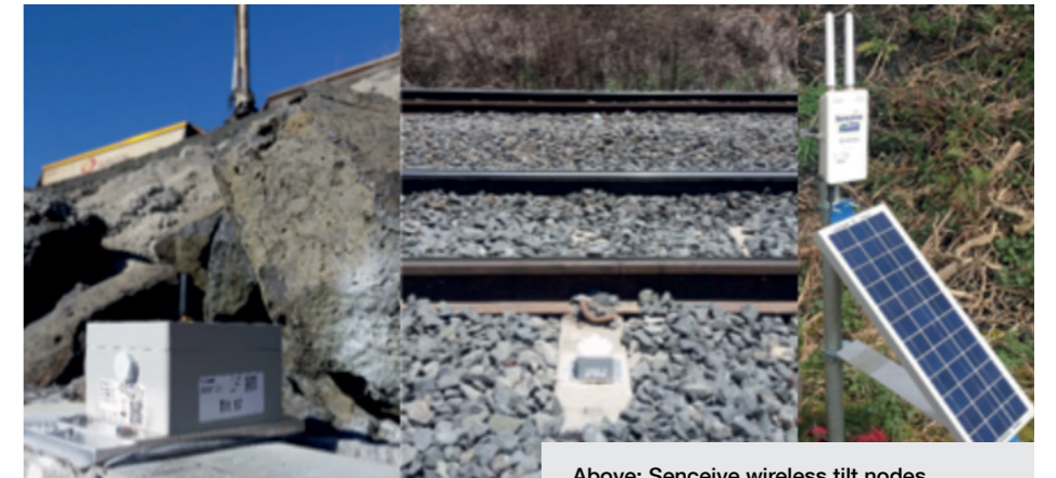
Above: Senceive wireless tilt nodes monitoring the rail track and a retaining wall. A solar powered 3G Gateway.
